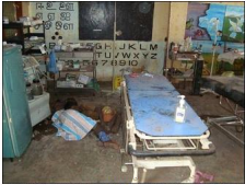
The makeshift Intensive Care Unit (ICU) sustained damage in the attack. Two dead patients. The makeshift ICU has been setup inside a class room of the school building.
